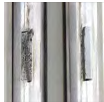
Damage to key from excessive wear
